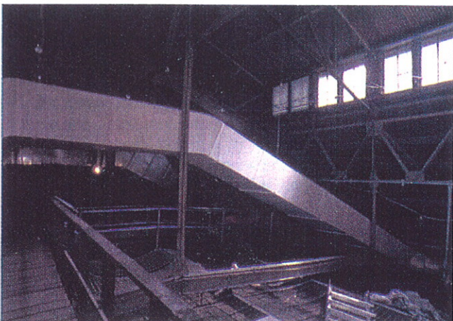
The new ductwork is located above the main historic concourse ceiling.
